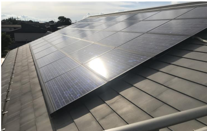
Photo 2: Solar panels at home
