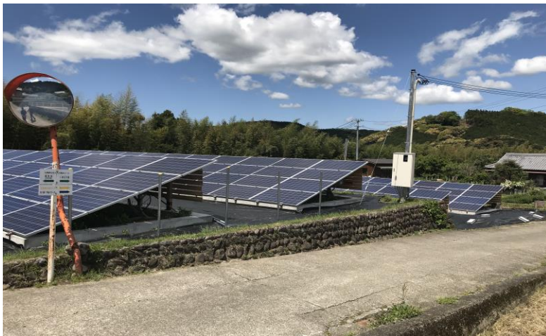
Photo 3: GPP (Green Power Partners LLC) No. 1 Power Plant located in Kamitonda, Tanabe City, Wakayama Prefecture
